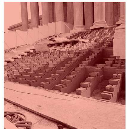
Supreme Court west terrace and steps renovation. Though a separate branch of government, the Court relies on the AOC to help maintain and modernize its buildings. Loretta Beasley, 10.1.1991
