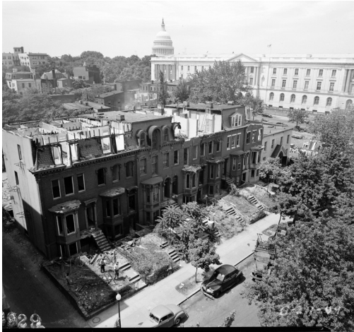
View from the top of apartment house on the north side of C Street, NE showing start of demolition of row of houses to make room for Additional Senate Office Building (later named the Dirksen Senate Office Building). Large format black and white film — geometry, detail, archival durability. Harry Burnett, 6.27.1949
