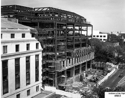
Hart Building under construction, steel superstructure near completion. Site addresses the Dirksen Senate Office Building and leaves space for the historic Sewell House. Harry Burnett, 7.27.1979
