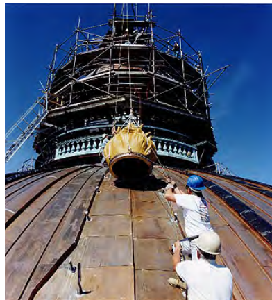
Reinstallation of the gilt copper flame atop the Thomas Jefferson Building, Library of Congress, part of a holistic renovation of the building that included the conservation of dozens of fine art murals decorating the inside of the building. Chuck Badal, 6.23.1997
