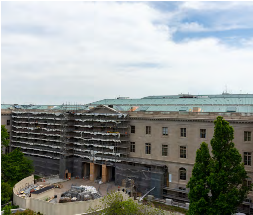
▼ Left: Scaffolding and construction site for the Russell Exterior Envelope Project. Right and Bottom Photos: Employees of the AOC Construction Division are shown building the Capitol Grounds and Arboretum storage shed.
